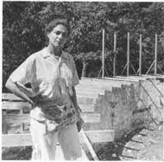
Mary Miss checks construction of walkway that follows the east edge of the old swimming pool. (photograph by Robert LaRouche, courtesy of the Post-Dispatch )
